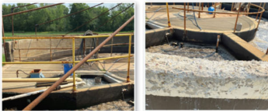
Medford Wastewater Treatment Facility
